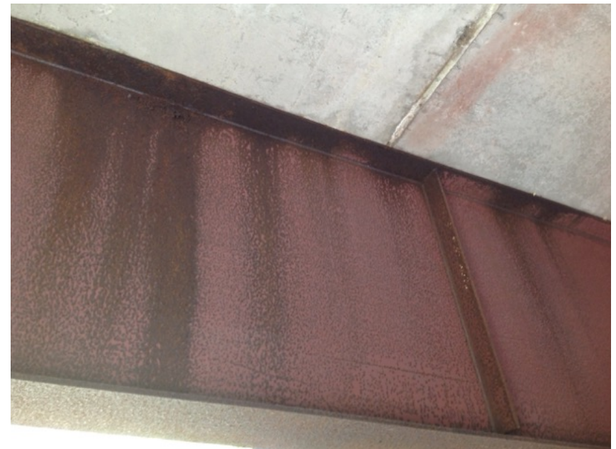
indication that moisture is getting through deck joints
