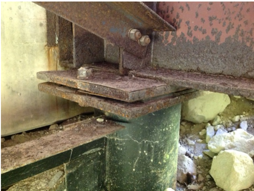
bearing plates delaminating - typical right bank
